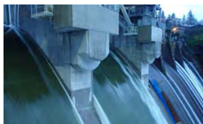
Flow from new Spillway Gates No. 1 and No. 2. Remaining old spillway gates can be seen in the background.
