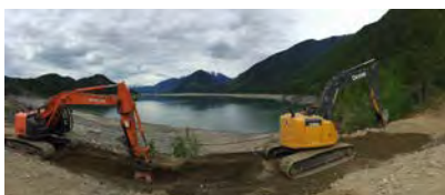
Duncan Dam- Preparation of the site prior to installation of the sheet-piles
