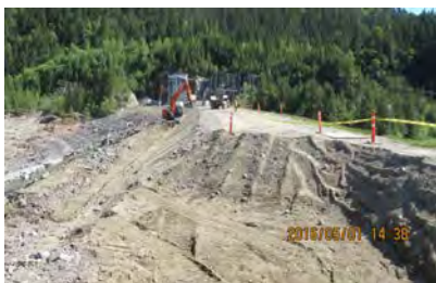
Duncan Dam- Preparation of the site prior to installation of the sheet-piles
