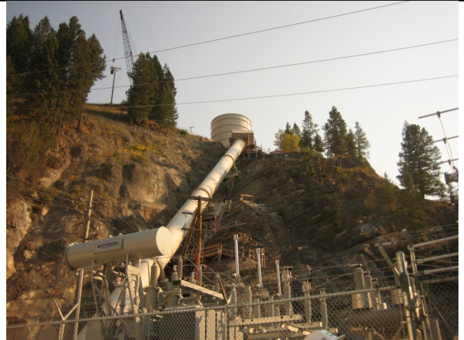
New steel penstock and surge tower
