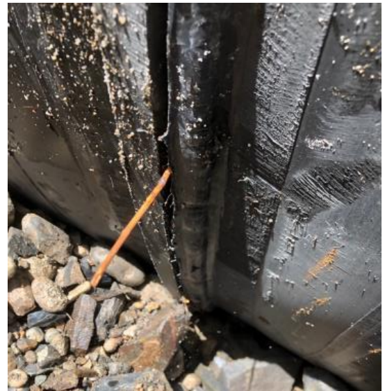
Figure 5 Weld failure at elbow joint observed after excavation.
