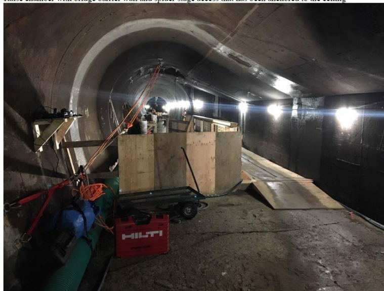
Raise chamber with bridge barrier wall and spider stage access that has been anchored to the ceiling
