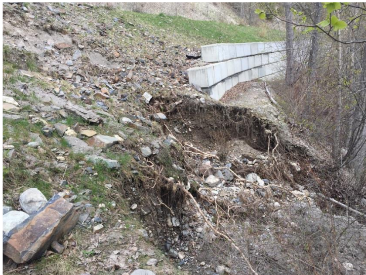
Figure 4 Erosion of the penstock slope above the road. The penstock is buried under the fill to the left of this photo.
