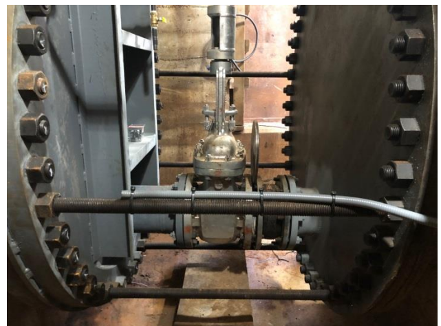
Figure 4 Blocking flanges and bypass valve installed to replace the damaged penstock intake valve at Spillimacheen.
