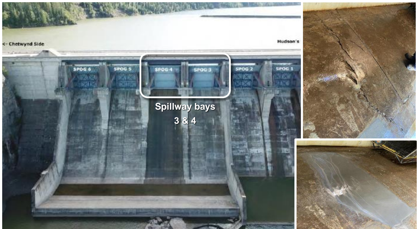
Figure 7 Peace Canyon Dam spillway concrete repairs: (Left) Location of repairs; (Upper right) crack in bay 3 between stoplog and spillway gate sills; (Lower right) repaired crack.
