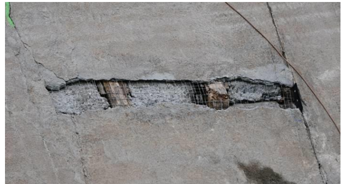
Figure 15 Large repair area chipped open and exposed on the face of La Joie Dam during this year's annual maintenance.
