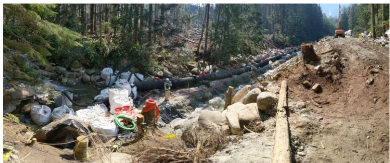
Figure 6 Water diversion in place at Boulder Creek and rip rap placement occurring at the dyke toe.
