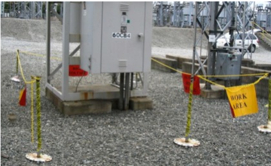
Plastic chain barrier using on-site fabricated steel stanchions
