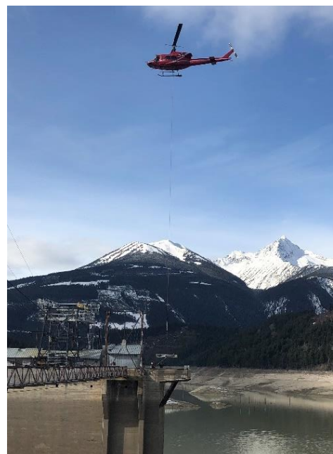
Figure 8 Delivery of new Intake Operating Gate 4 followers to intake deck at La Joie Dam.
