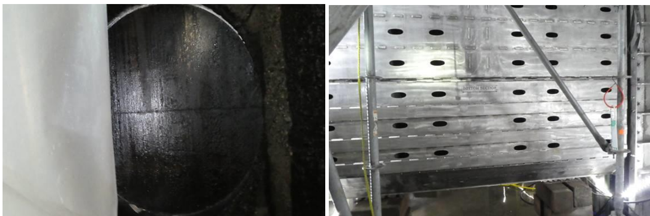
Figure 7 Downstream side of old intake maintenance gate (left) and upstream side of new intake maintenance gate (right).
