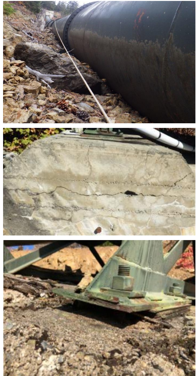
Figure 6 Bridge River 1 penstocks: (top) accumulated rockfall covering foundations and portions of penstock; (middle and bottom) damaged penstock foundations.
