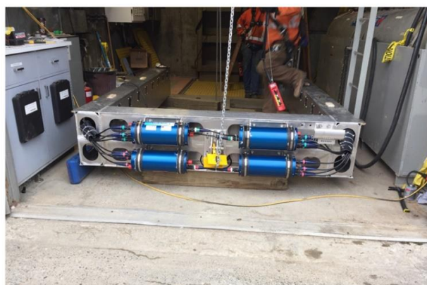
Figure 9 New over velocity detection system at Wahleach on its mounting frame.
