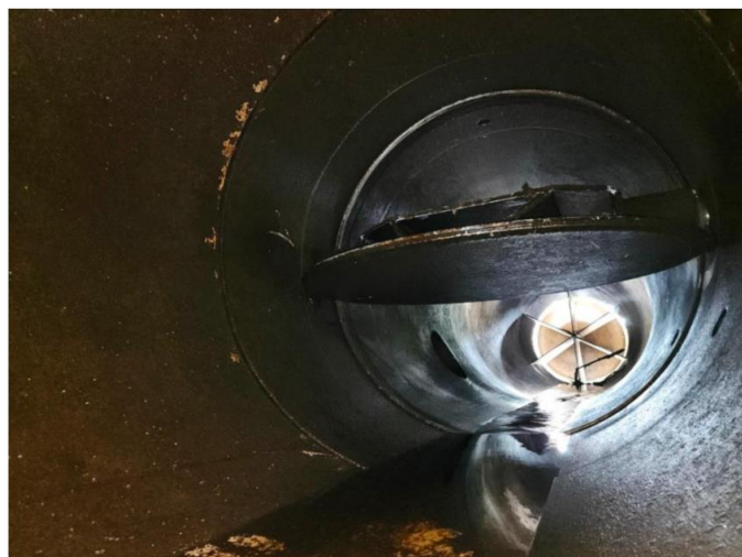
Figure 5 Ash River low level outlet, looking downstream with the butterfly valve in the foreground and the hollow cone valve in the background.
