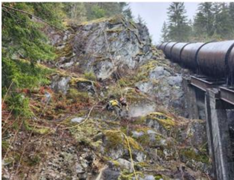
Figure 7 Scaling and meshing in progress at the trestle section of the Cheakamus penstocks.
