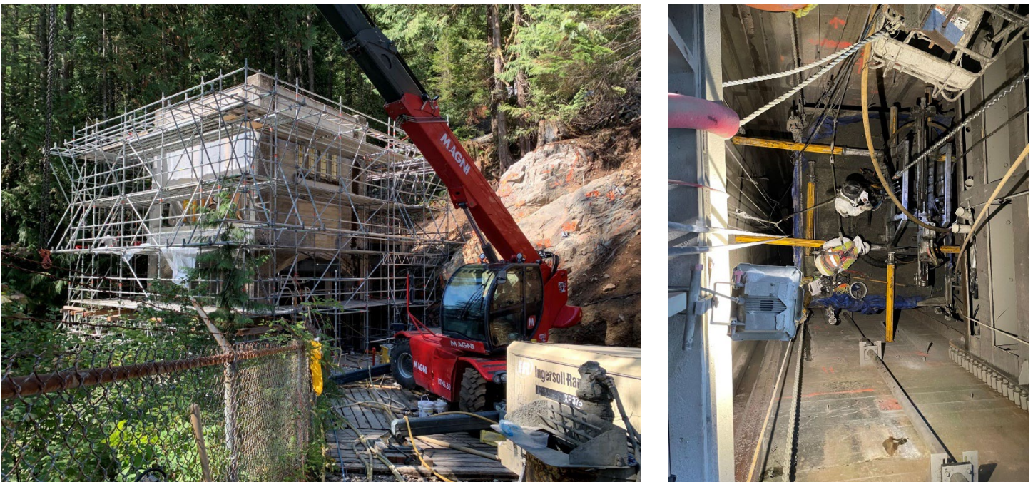
Figure 7 Seismic upgrades underway on the structures of the Alouette Tunnel. At left: surge tower superstructure. At right: surge shaft concrete lining; work being performed from suspended platform that is raised and lowered along the shaft as required.
