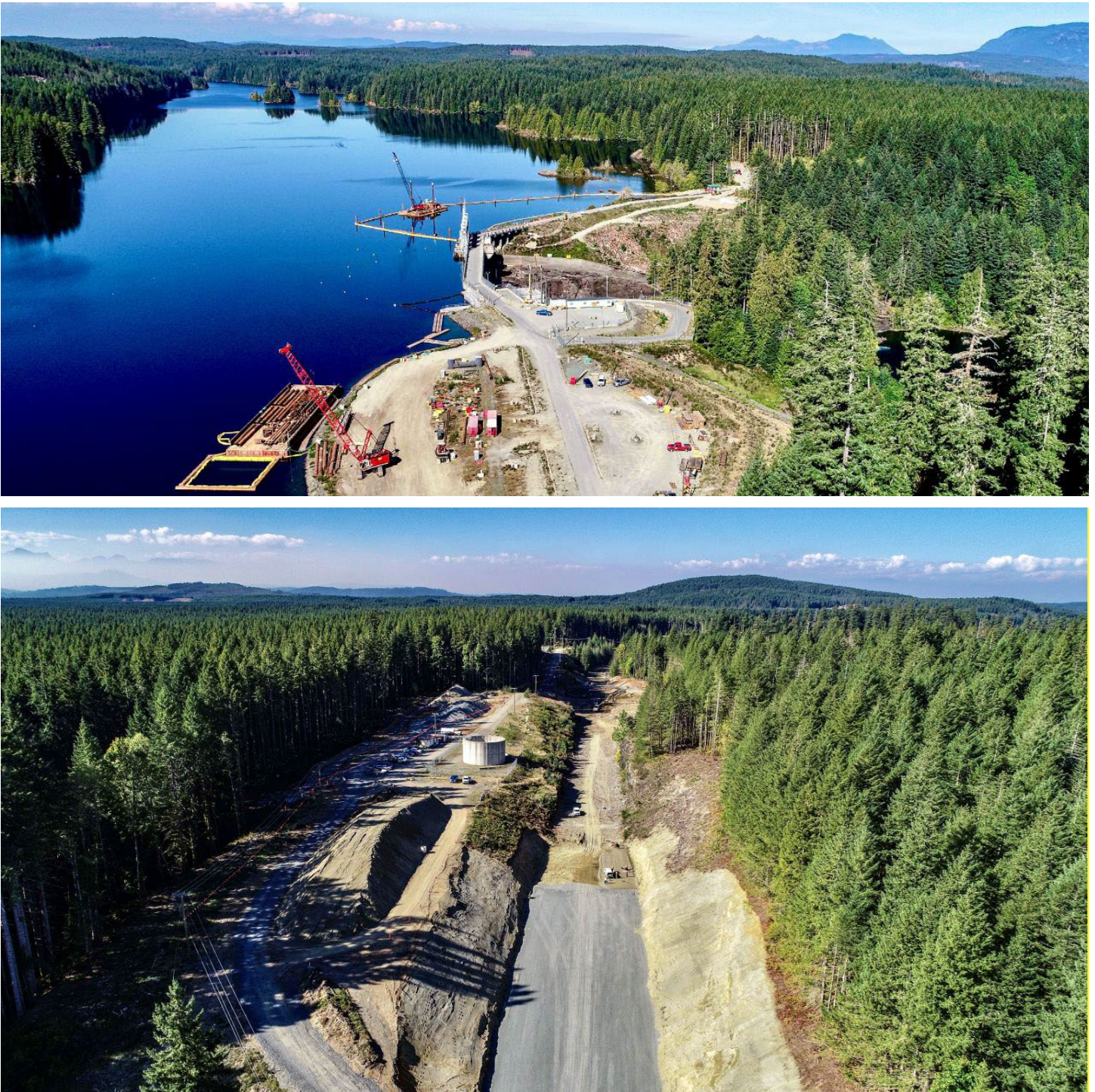
Figure 9 Construction on the John Hart Dam Seismic Upgrade Project is underway, as seen in these September 8 photos from the site. Top: Work area on the Middle Earthfill Dam (foreground) and installation of the silt curtain upstream of the North Earthfill Dam (background). Bottom: Construction of one of three containment berms along the old penstock corridor, where dredgeate from the reservoir will be placed.
