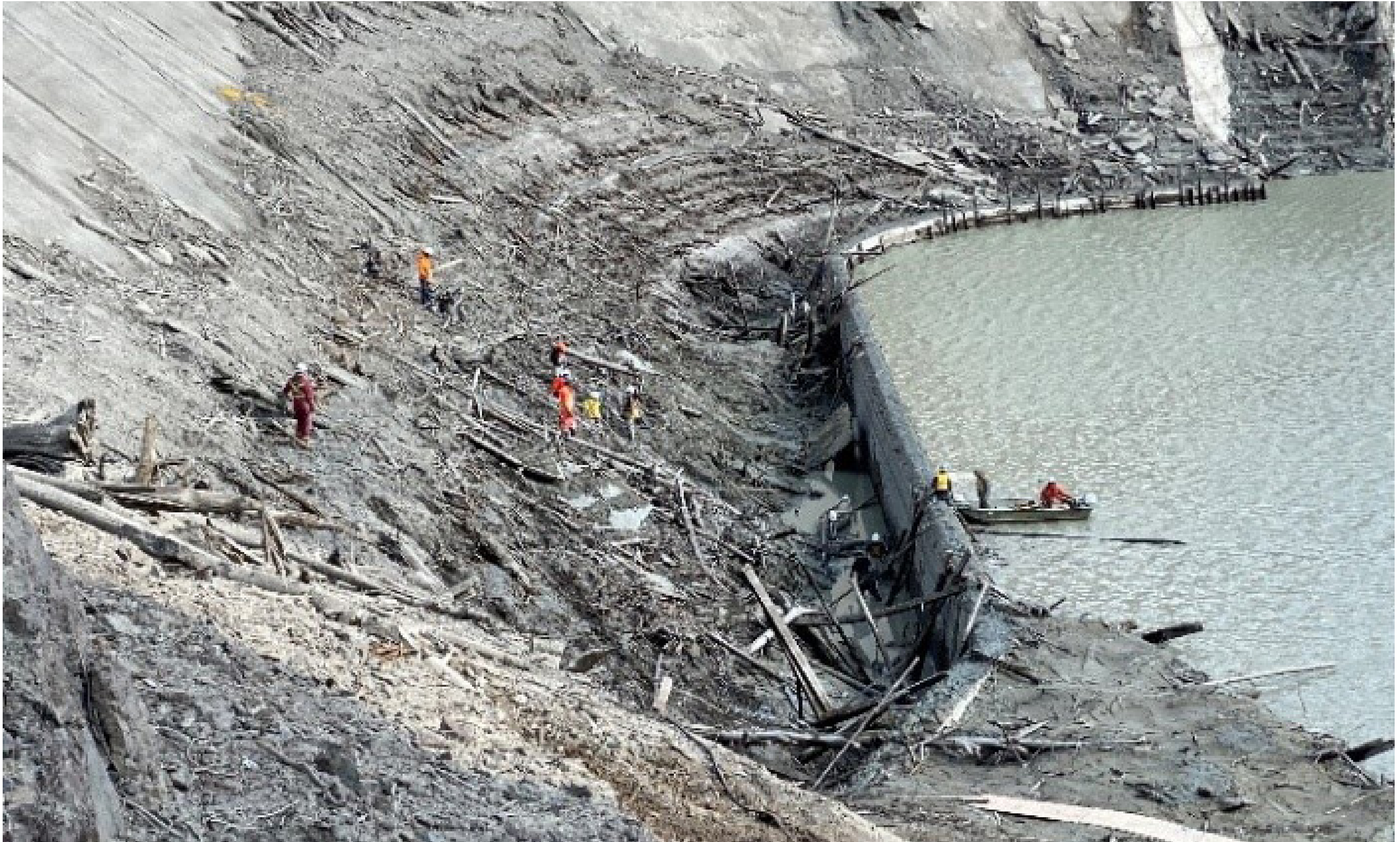
Crews investigating at the toe of LaJoie Dam during the April 2022 drawdown
