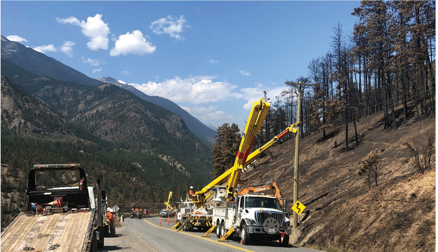
BC Hydro crews work along Highway 12 to restore infrastructure impacted by a wildfire. Photo credit: Ryan Micholuk.
