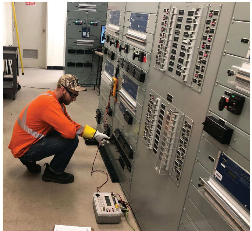
Kyle Douglas performs a load test at the Bridge River 2 Generating station. Photo credit: Sean Baylis.
