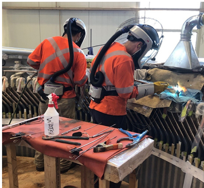
Winders brazing copper coil connections. Oxygen/acetylene torches were used with extreme caution.
