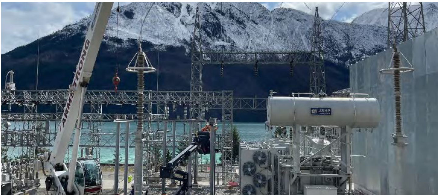
Crews install steel components in late March as part of the Transformer 3 Replacement Project at Bridge River 1. The project is expected to be completed this summer.
