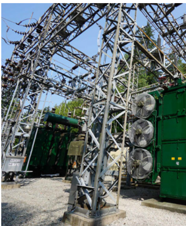
Existing substation inside the fence
