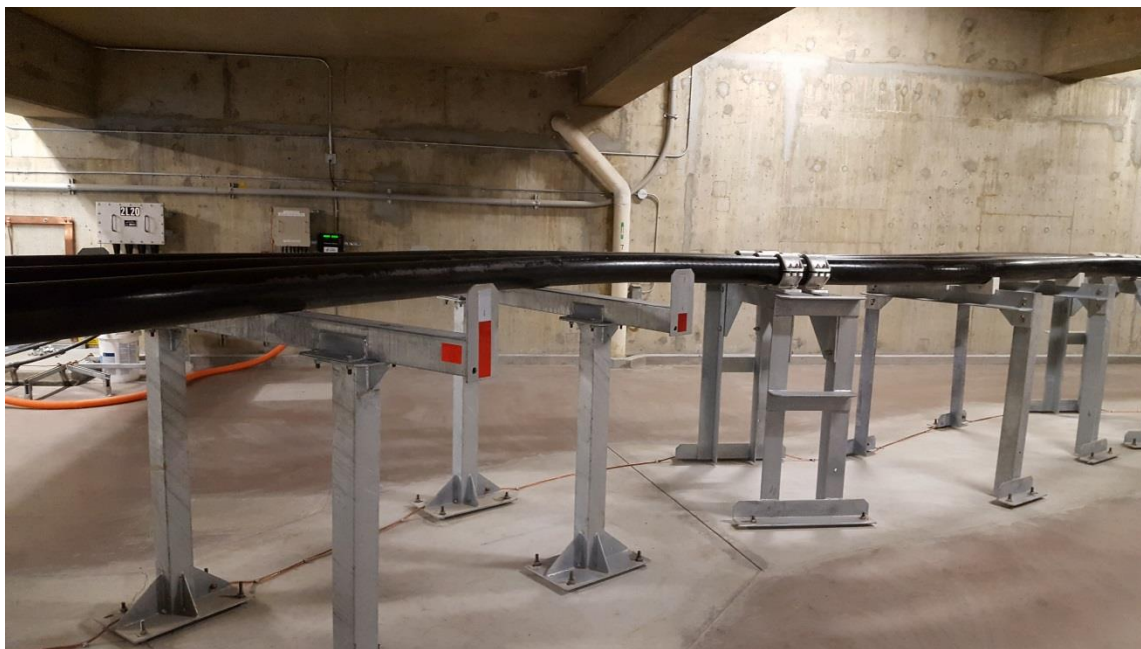
Figure 3: Measurement location near 2L020 (230kV Cables) inside CSQ Substation, Level 1.
